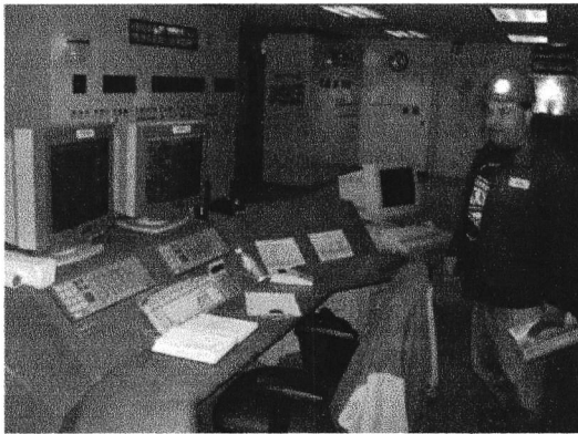
Left: One of the control rooms.
